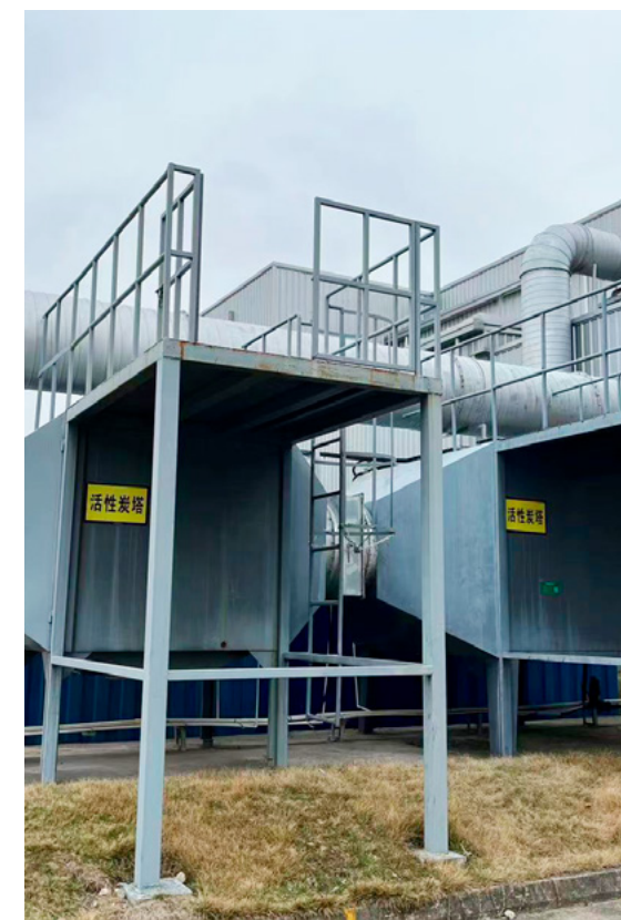
Double activated carbon facility at GC Suzhou
